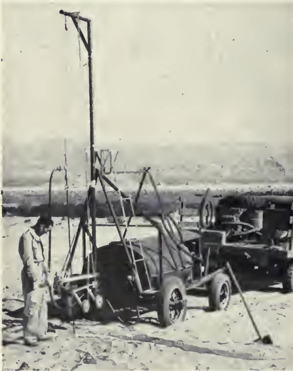
THE PROBE —At top, the hydraulic rotary drill and coring rig used to extract samples and dig observation wells at 42 sites in Coachella. Below, a Coachella Valley County Water District employee installs a piezometer by means of the jetting process. Top photo submitted through the courtesy of the United States Salinity Laboratory, Riverside, Calif.
